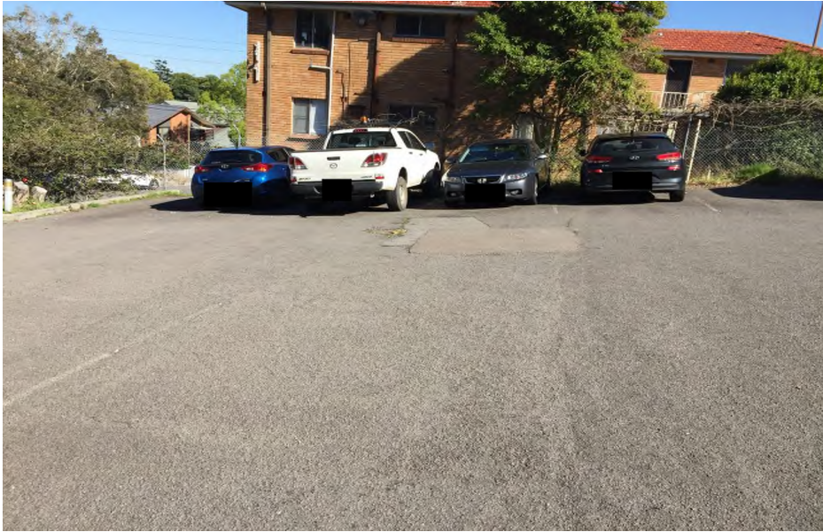
Photo 5: Asphalt surface condition in car park
