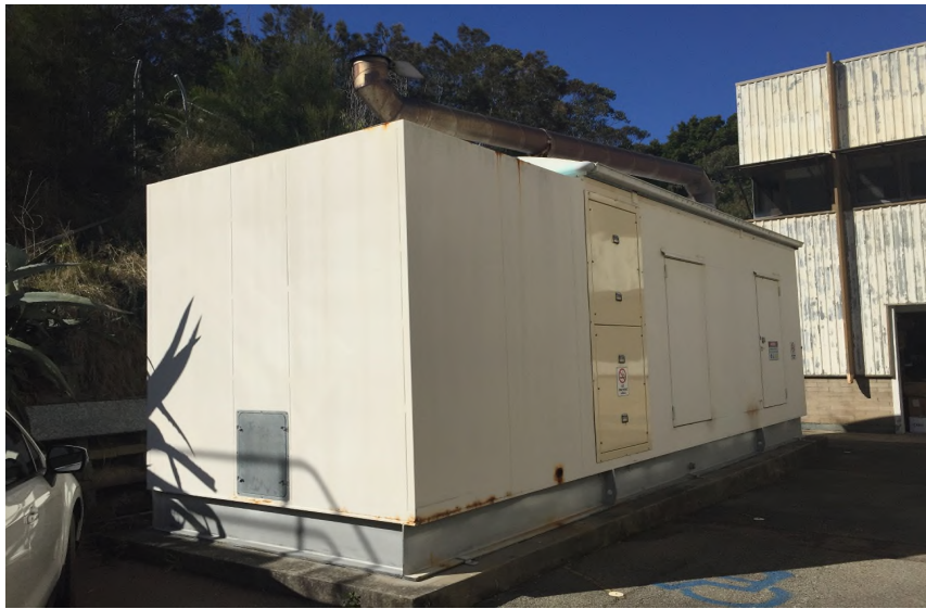
Photo 11: Stand-by generator located in the eastern section of the Site
