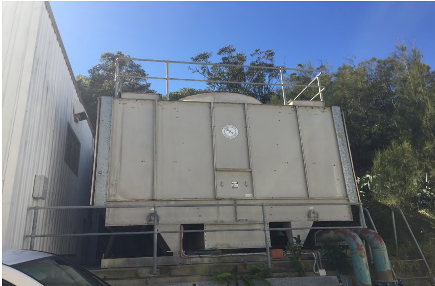
Photo 7: Cooling Tank on the eastern portion of the Site
